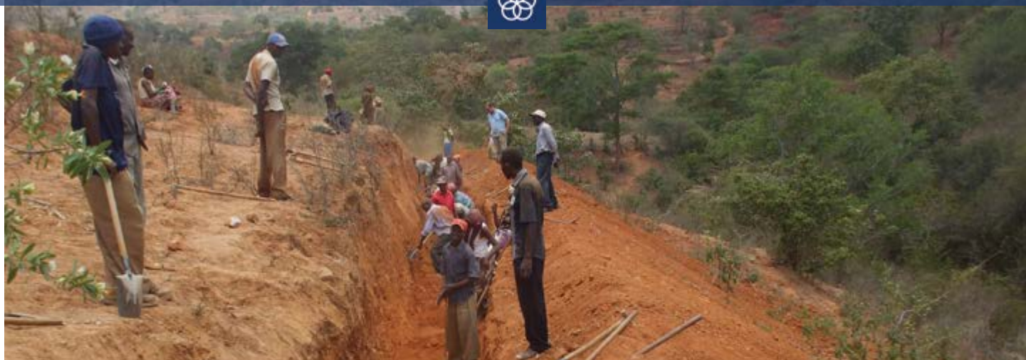
Prairie Wind Mennonite Church: Ngaa community members laying terraces on sand dam banks as part of Prairie Wind Mennonite Church's 'Self-Help Group Water Project' in Kenya.
